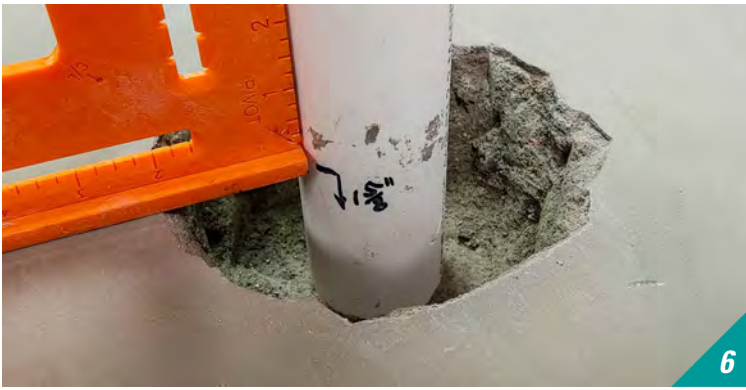
Using a speed square and permanent marker, mark the exact slab elevation on the pipe.
