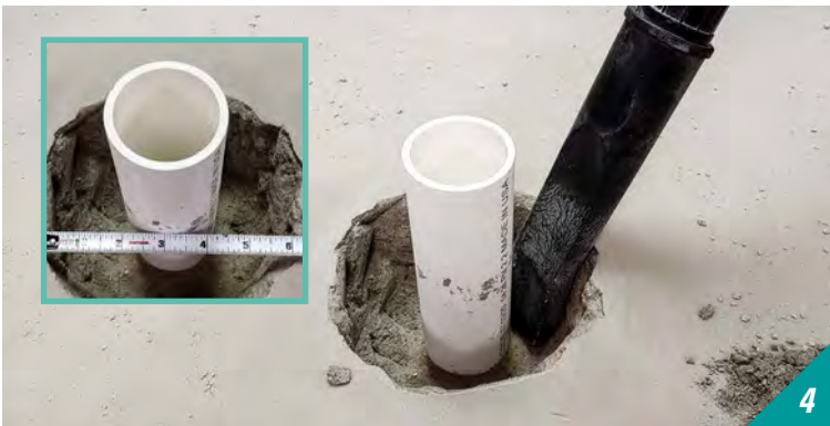
4 Continue breaking the concrete around the pipe and remove debris as needed with a shop vac.
