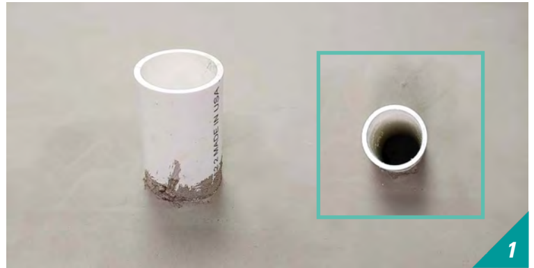
1 Ensure the concrete slab in the shower pan area is level. Use SLU as needed to level the shower pan area.
