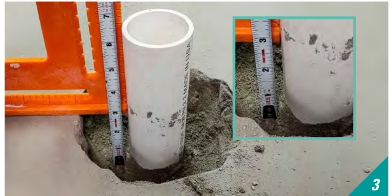
3 Using a speed square and tape measure, continue to dig out the depth of the hole around the pipe. The recommended depth is 3" while the recommended diameter range is 5 ½" to 6 ½".
