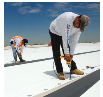
JM’s roofing system provides a weathertight environment for this grocery service distribution center in Colorado.
